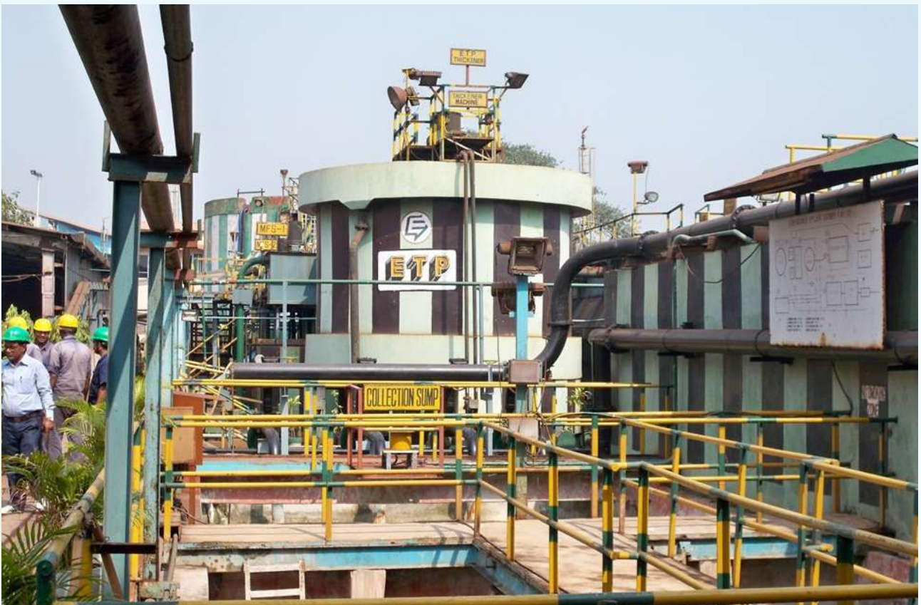
Figure 3 - Common Effluent treatment plant at Khardah
